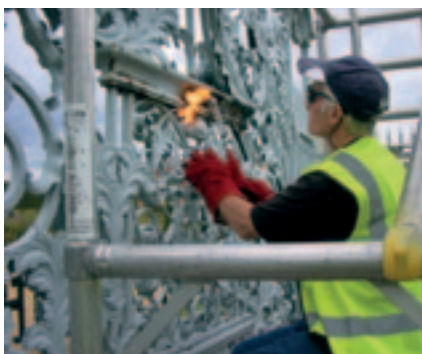
Adrian Wolfe, an NHIG student, flame cleaning a section of the Hampton Court screen to expose the condition of the underlying metalwork (Photo: Bethan Griffiths)
