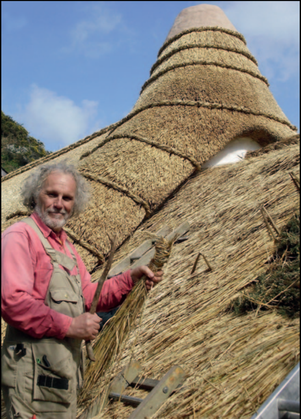
Alan Jones stuff-thatching threshed long straw into a base coat of gorse at Llanon, Dyfed: this rare example of the west Wales vernacular is supported by a thick mat of twisted straw rope across the purlins, and includes a thatched chimney. Photo: Wilm Jones, Pembrokeshire Thatch & Carpentry Services
