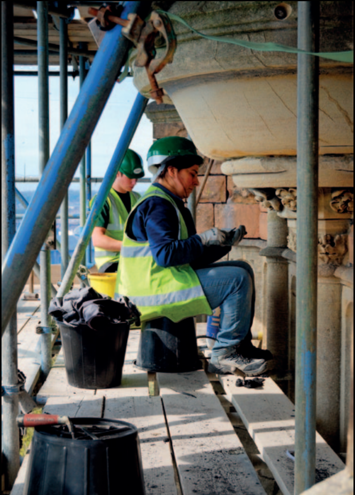
Nimbus Conservation conservators at Cabot Tower, Bristol: the heavily eroded mortar joints are being repointed with a hydraulic lime mortar coloured with coal dust to match the original. Photo: Jonathan Taylor
