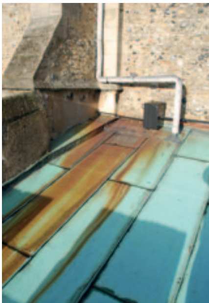
Iron-staining caused by a steel overflow pipe to the heating system
