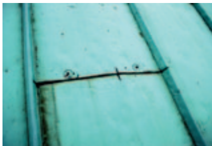
Chichester Cathedral: the wide bays used between vertical seams allow the sheet to deflect under wind-lift which can cause hardening of the metal and eventual cracking.
