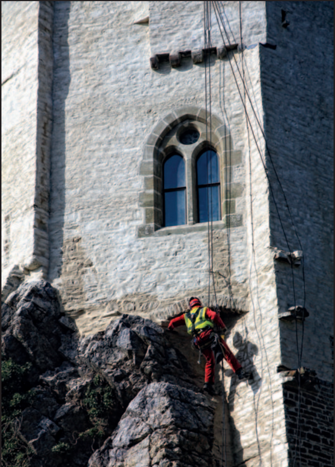
Applying a hydraulic lime shelter coat under challenging access conditions at Roch Castle, Pembrokeshire (see article, page 13) Photo: Acanthus Holden Architects
