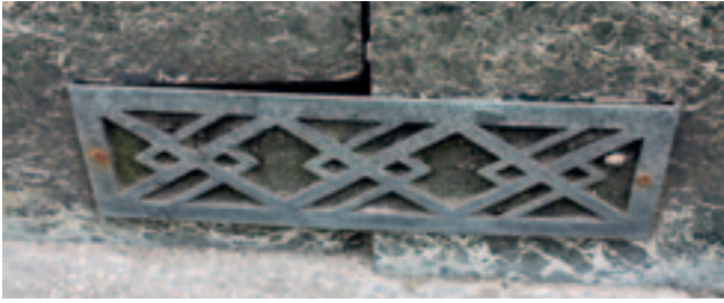
Bronze stall-riser vents set in green marble: These small details are important. Bronze vents varied in style but were always integral to the overall design. Damage to the marble is also evident.
