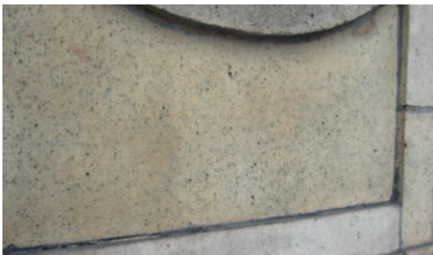
Sandblasting of terracotta units often leads to a pitted surface. Due to the temperature and duration of firing, the internal body of the block is still resilient to weathering. (All photos on this page: Steven Handforth)
