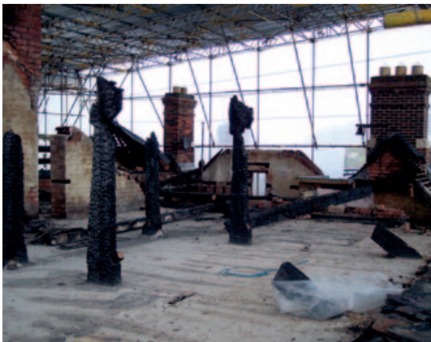
The floor of this fire damaged building was found to be constructed of reed and lime plaster. Failure to expose the underside had promoted mould growth, and further remedial treatment was required to promote drying prior to decontamination. (Photo: Hutton + Rostron)
