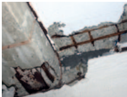
Typical corrosion of floor slab reinforcement
