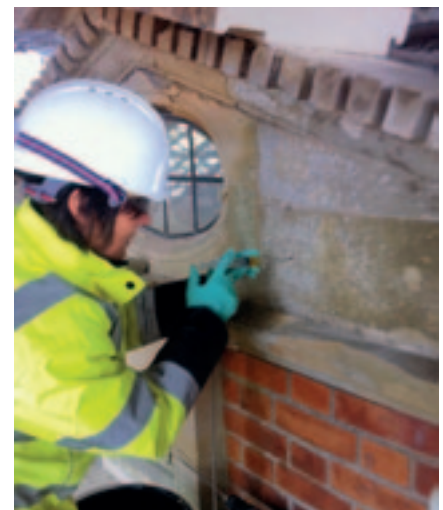
Jackie Blackman, a student from City of Bath College preparing to insert a stainless steel rod to fix gable masonry at the Tyntesfield orangery for her NVQ level 3 (Photo: Nigel Bryant)
