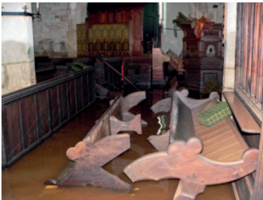
The church interior as the waters receded with the high water mark clearly visible on the wall
