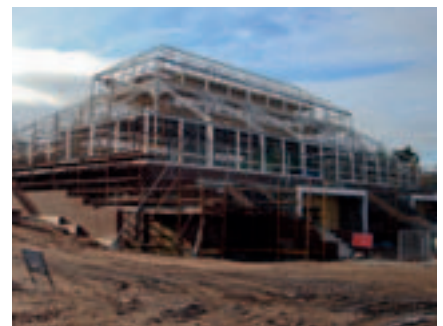
The wrought and cast iron frame was carefully recorded and dismantled for restoration off site in workshop conditions. This allowed the construction of the contemporary basement structure which would provide a café for the park and all ancillary accommodation. The restored frame was then re-erected on its new base.
