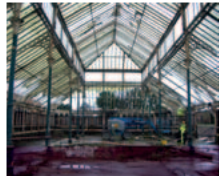
Prior to the regeneration the conservatory was a ruinous shell.
