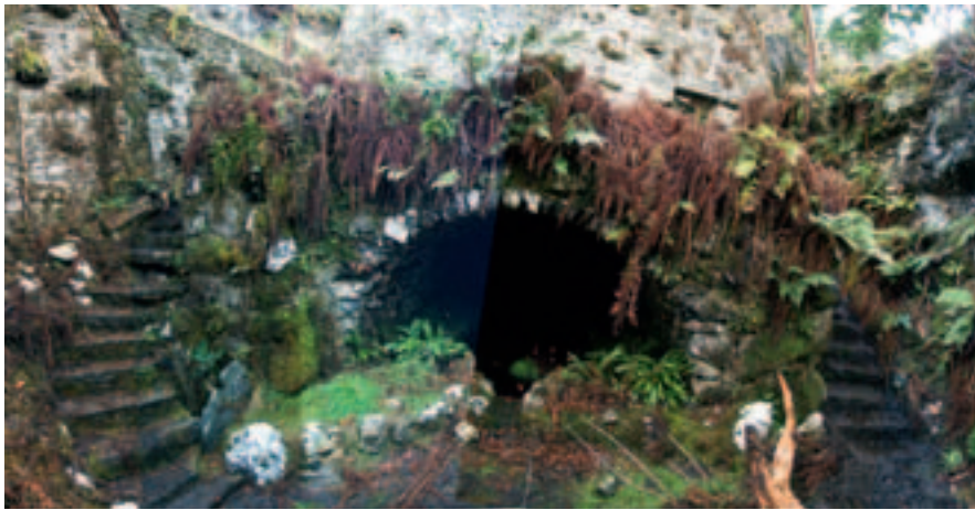
The grotto and stairways before conservation (Photo: MAST Architects)
