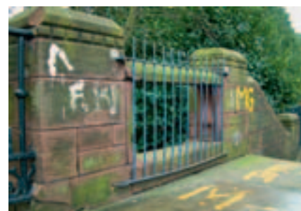
Typical damage to the stonework baluster detail to the abutments of the composite bridges
